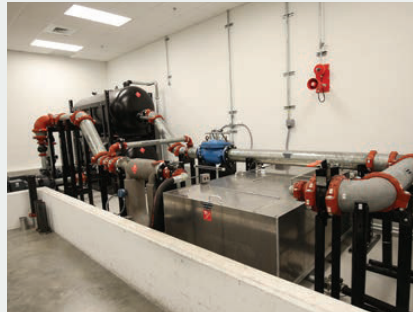
FUEL FLOW METER TEST STAND
