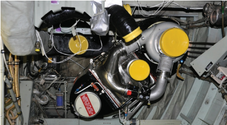
New ECS Refrigeration Unit
